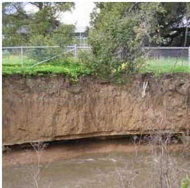
Example of creek bank erosion.
