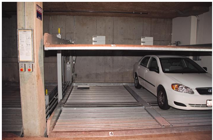
Photo 4-1. Parking Lifts in Parking Garage, Berkeley
