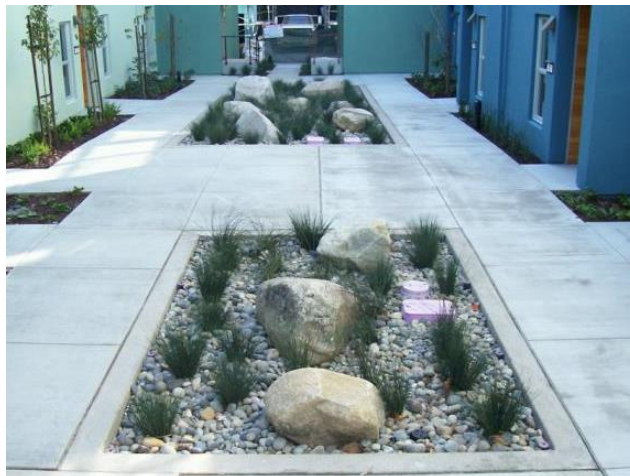
Photo 8-2. Flow through planter in the City of Emeryville
